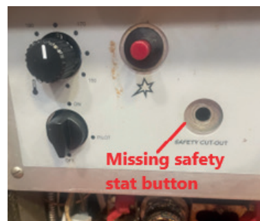
Gas fryer – safety stat reset button damaged/missing.
